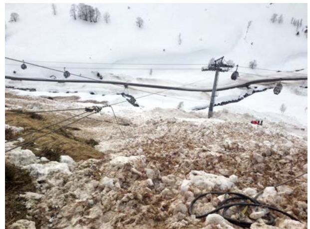
Figure 9. View of the tower taken from above on 18 February 2013. A wire was stretched to stabilize the tower pushed over by the sliding slab. Courtesy of J.-L. Pons.
